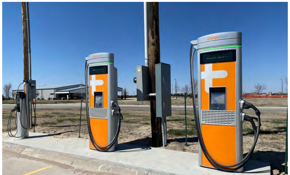
Electric Vehicle Charging Stations, Hebron Source: Marvin Planning Consultants
