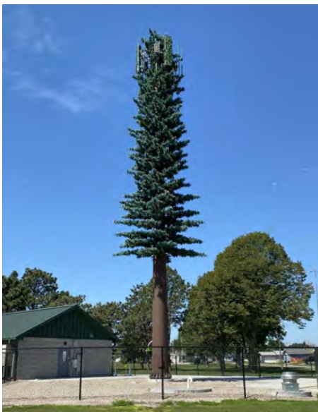
Stealth Cell Tower Source: Marvin Planning Consultants
