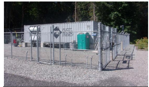
Example of a standalone BESS Facility Source: American Planning Association
